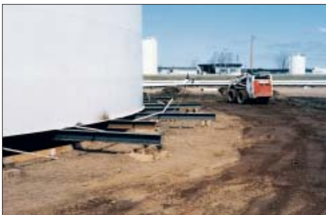
Here are two examples of major tank repairs: a man-way installation (top) and elevation ("jacking") of an entire tank shell.
