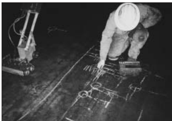
MFE scan has indicated soilside metal loss (Fig. 5).
