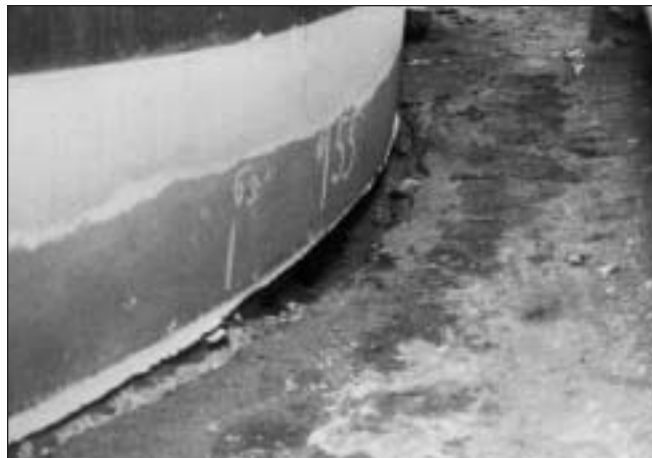
Exterior tank inspection has turned up bottom sketch-plate deterioration (Fig. 1).
